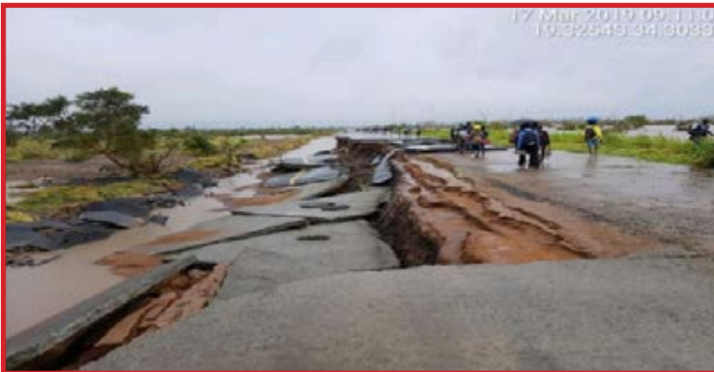
Image 7: Damaged communication route in Sofala Province. Source: INGC
