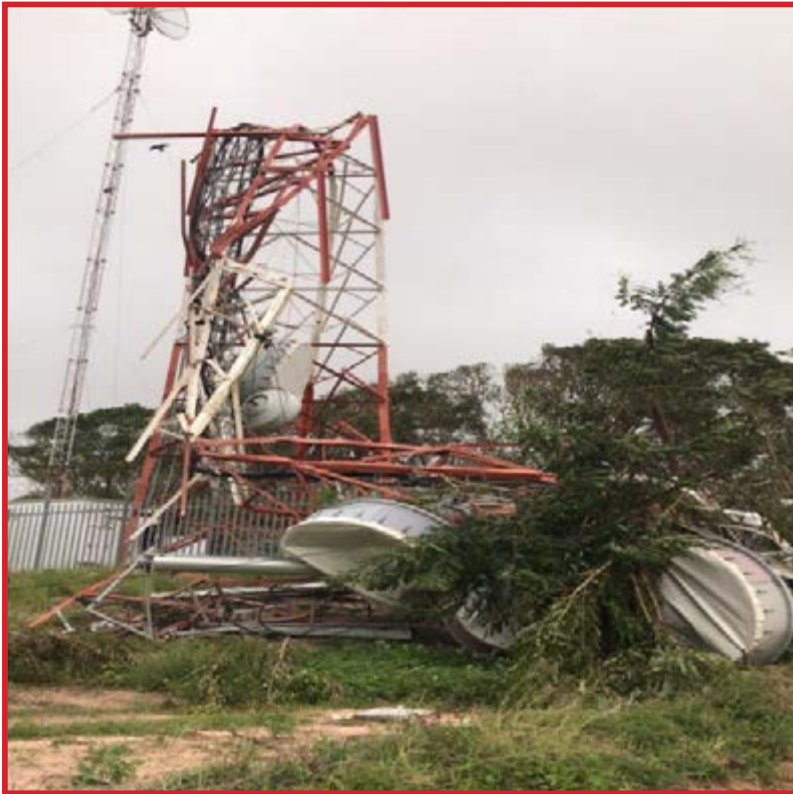
Image 6: Tmcel operator's damaged tower in Sofala Province. Source: INCM
